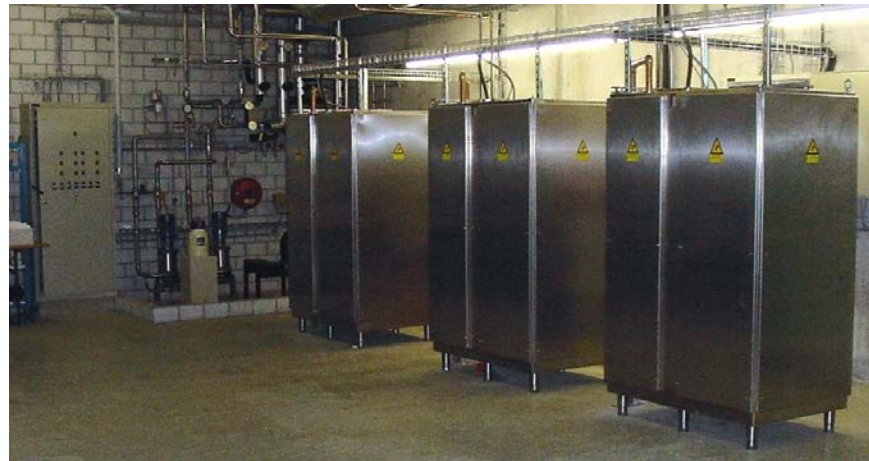
3 x 30kW 27.12MHz RF generators (GHP300KE, Sairem) and their water cooling circuit in an induction heating application
